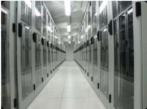
Gambar 2. Dedicated Server dalam Data Center ( http://sites.google.com/a/kainoshealth.net/syncmed-healthcare-solutions/Home/Data-Center-Specifications/datacenter.png )
